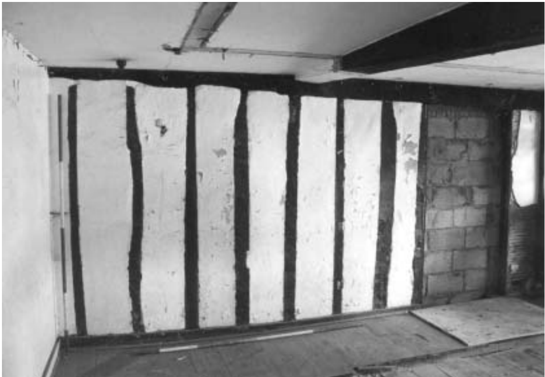
Plate 12 Timber-framing on the internal NW wall of the first floor of Building C
